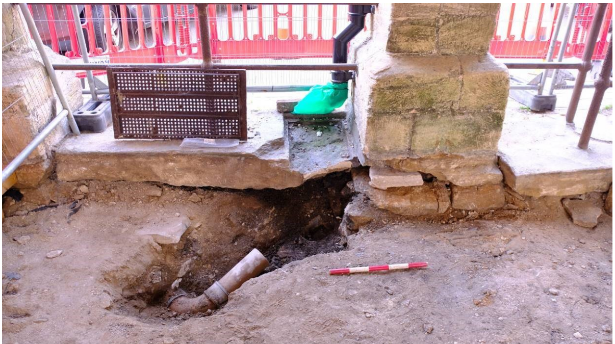
Fig. 18 View of drain in Southwestern corner of undercroft showing undermining of pier base (looking west, scale 0.5m)
